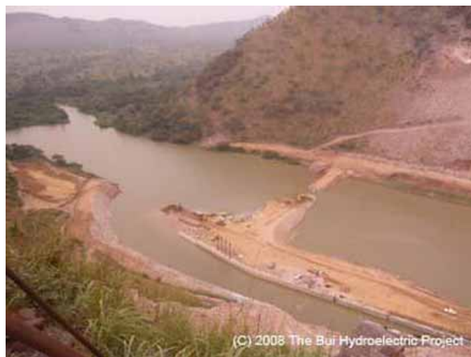
Diversion of the Black Volta River for the Bui Hydroelectric Dam Project
